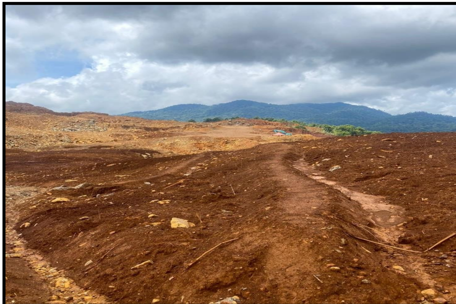
Figure 11 Actual contour drain at Konde Central Pinnacle
